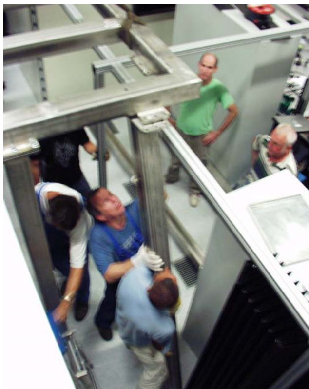
Figure A.5: During the construction laser work has to stop, so speed is of the essence.
