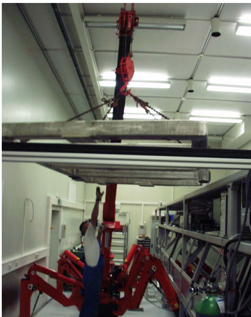
Figure A.2: Lifting a few hundred kilogram of steel frame above a sensitive high-power laser system.
