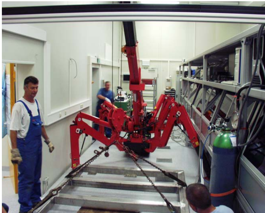
Figure A.1: The crane is ready to install the beamline in the cleanroom.
