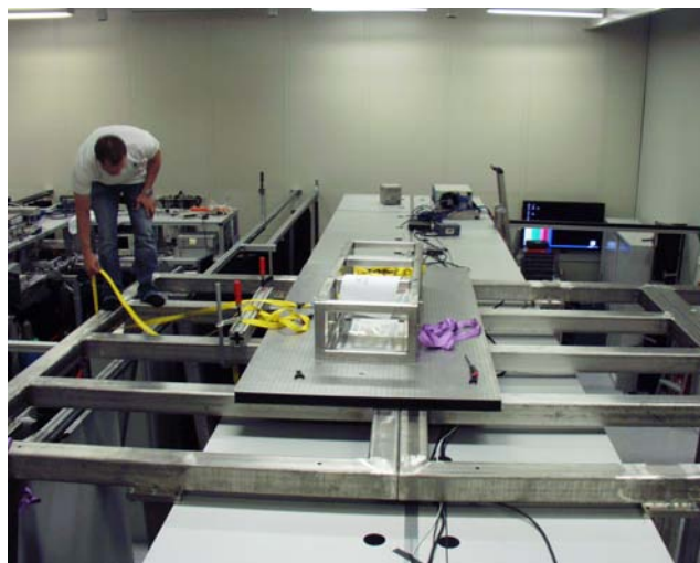
Figure A.9: There is still a lot of work left, but at least the basic fundament for the new high-flux XUV beamline AS 6 has been laid!
