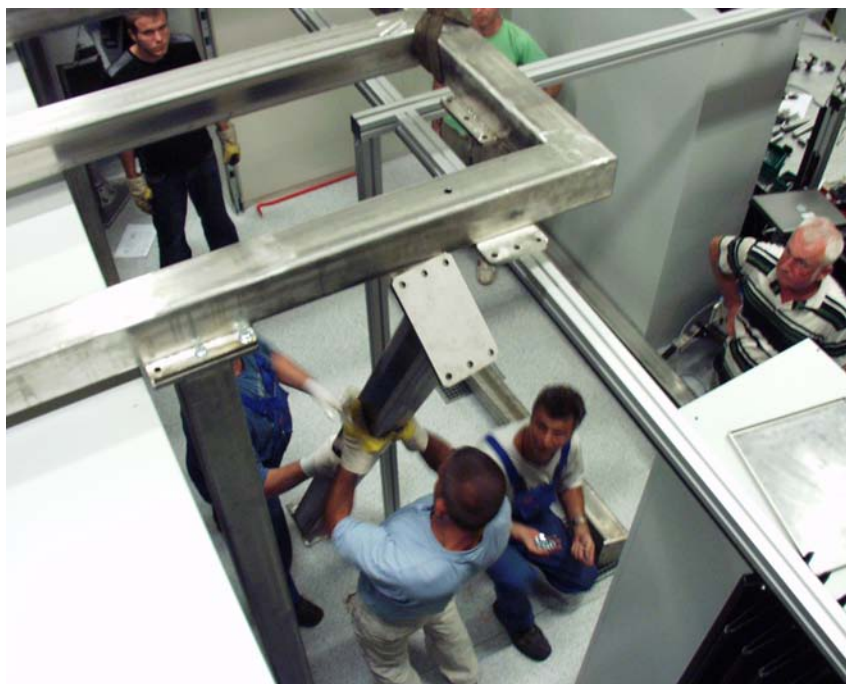
Figure A.4: To stabilize the bridge above the laser huge steel pillars are needed.
